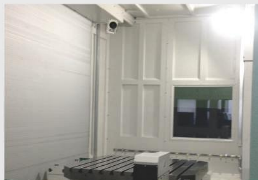
Fig. 04 Example of application of a flame detector
